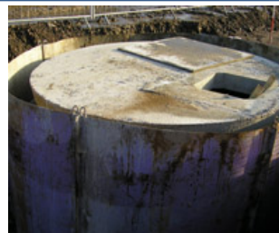
Traditional manhole surround
