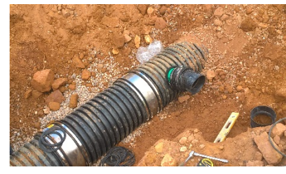
Plastic pipework making use of off cuts and bespoke gully tails
