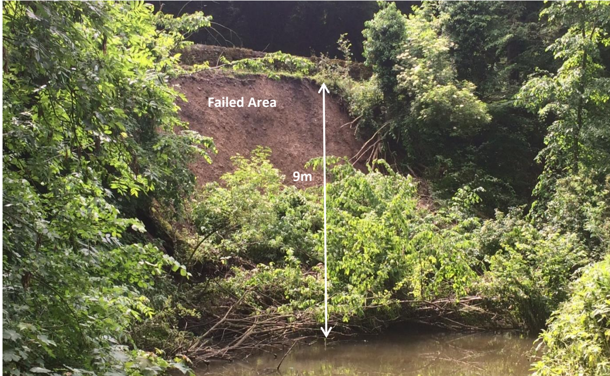
Figure 3 – View of Slope Failure
