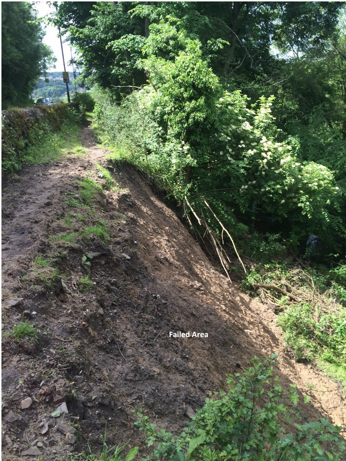
Figure 4 – Failure Viewed from Slope Crest
