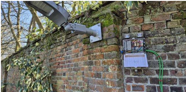
DC luminaire fed from a breakout box
