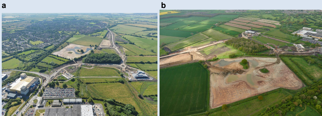
Figure 16: a) aerial view of the site (Derby City Council) b) flood alleviation scheme under construction (Derby City Council)
