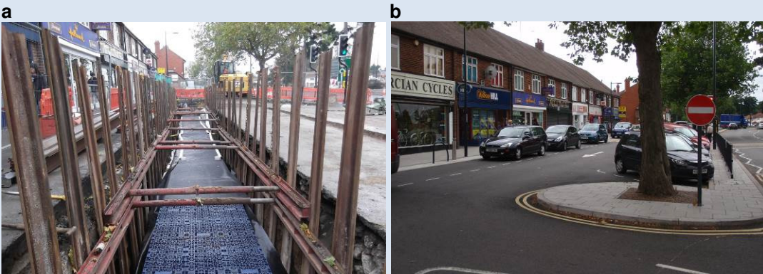
Figure 14: a) Storage tank construction (Derby City Council) b) Completed scheme (Derby City Council)
