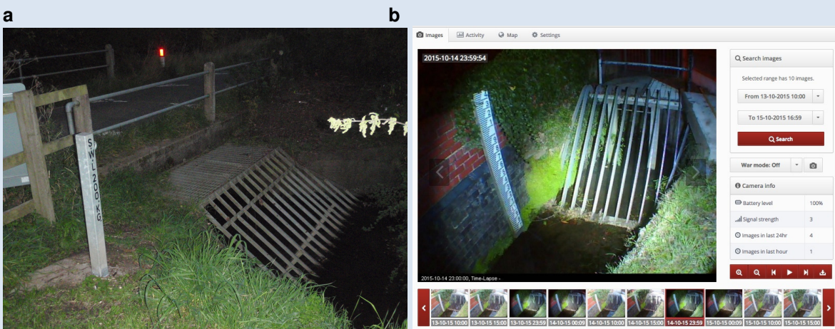
Figure 17: a) trash screen installed over a culvert (Derby City Council) b) CCTV image (Derby City Council)
