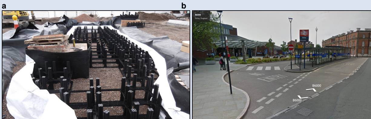
Figure 12: a) Storage tank under construction (Derby City Council) b) Scheme after completion (Derby City Council)
